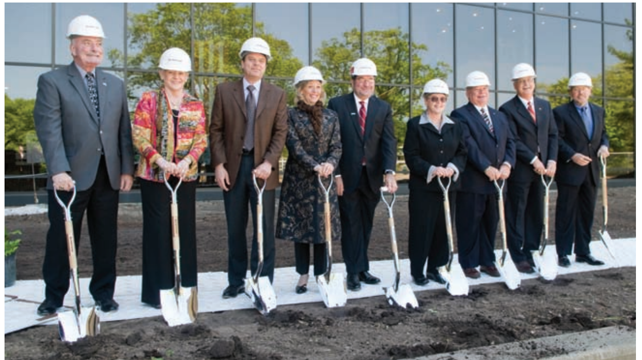
Representatives of MSU and major donors to Wharton Center’s capital campaign gathered on May 19, 2008, to break ground on the first major expansion and renovation of Wharton Center in its 25-year history. Pictured from left to right are: Larry Sierra, director of Intramural Sports; Arlene Sierra, assistant chair, Department of Radiology; Steve Roznowski, president and CEO of Christman Company; MSU Trustee Melanie Foster; Wharton Center Executive Director Mike Brand; MSU President Lou Anna K. Simon; MSUFCU President and CEO Pat McPharlin; Bill Latta, assistant director of MSU’s Office of Planning and Budgets and acting associate vice president of Advancement Services; and Jackson National Life Insurance CFO Andy Hopping.
