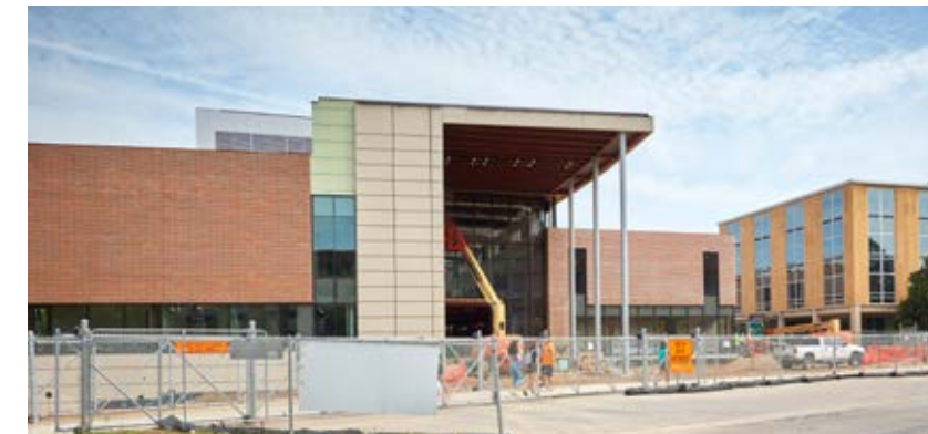
The Edward J. Minskoff Business Pavilion will connect to the North Business complex and Epply Center.
